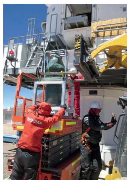
Figure 4. Installation of the DESHIMA cryostat (protected in a plastic bag) to the ASTE cabin.
